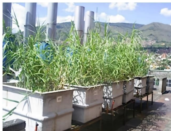
Figure 1. Subsurface flow pilot wetlands installed at the University Research Headquarters (SIU)
