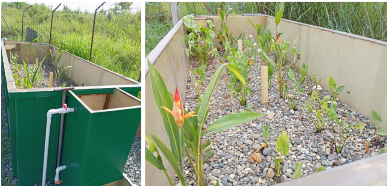
Figure 5. Pilot unit for the treatment of point source pollution using NbS
